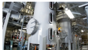
Aomori plant effluent treatment system
